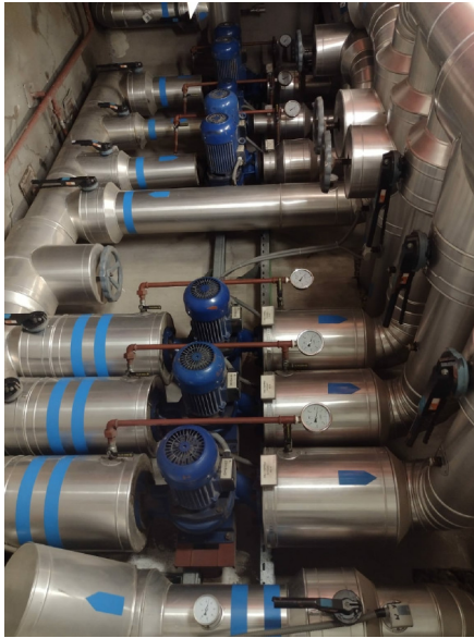
BOMBAS COLECTOR DE FRIO
